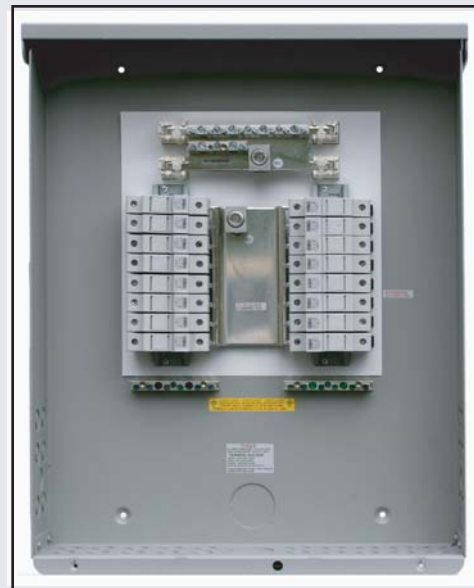
Busbar arrangement shown
