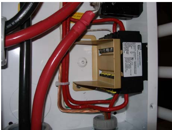
Din Rail mounted breakers
